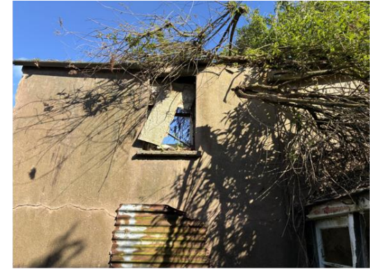
Plate 9: View of dilapidated structure during April 2026 survey
