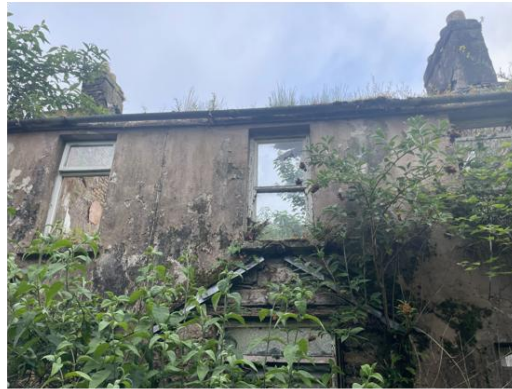
Plate 8: View of roofless dilapidated structure during May 2024 survey
