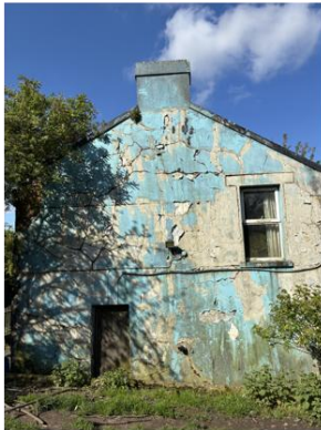
Plate 10: View of east facing gable end of the remaining dwelling on site
