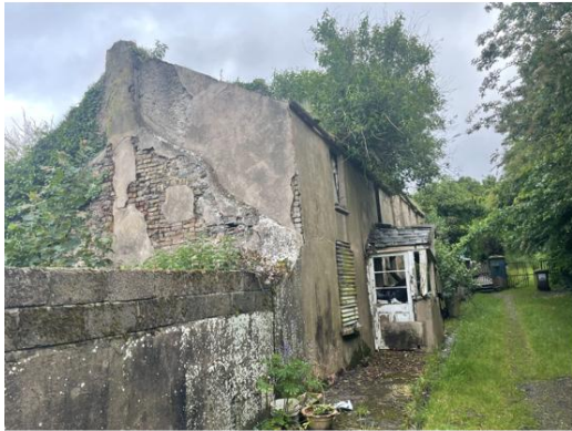
Plate 7: View of dilapidated structure at site entrance during May 2024 survey
